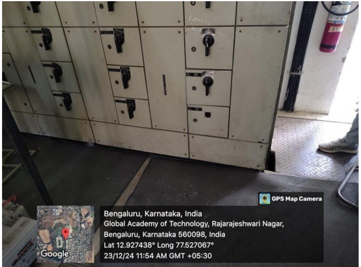
Figure 4-12: Electrical safety mats near electrical panel
