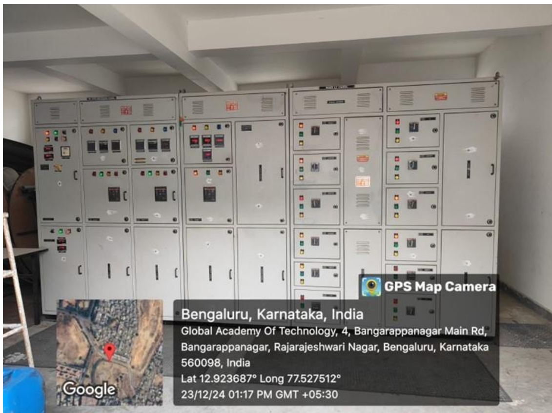
Figure 4-2: Electrical Panel room
