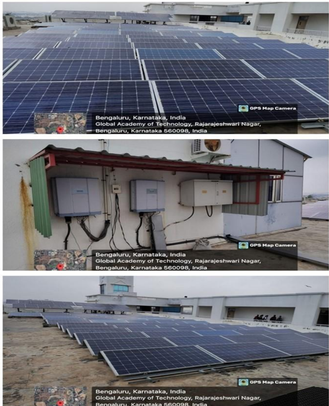
Figure 4-8: SRTPV installed at college
